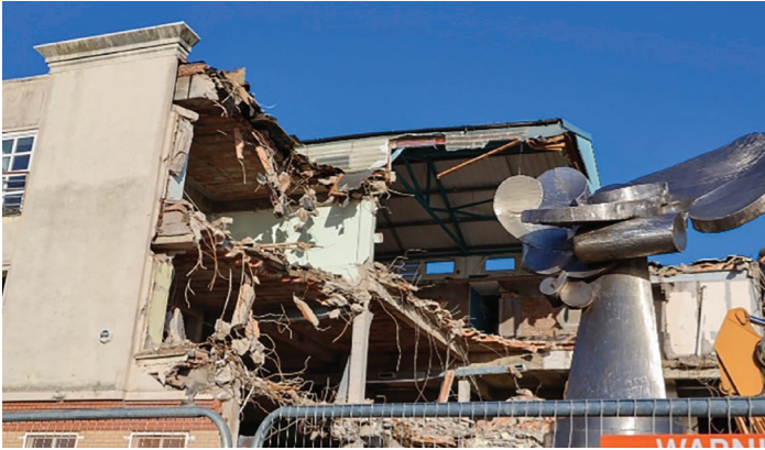
A farewell to familiar landmark buildings at the top of Drumchapel Shopping Centre... Picture: Kevin Harvey
